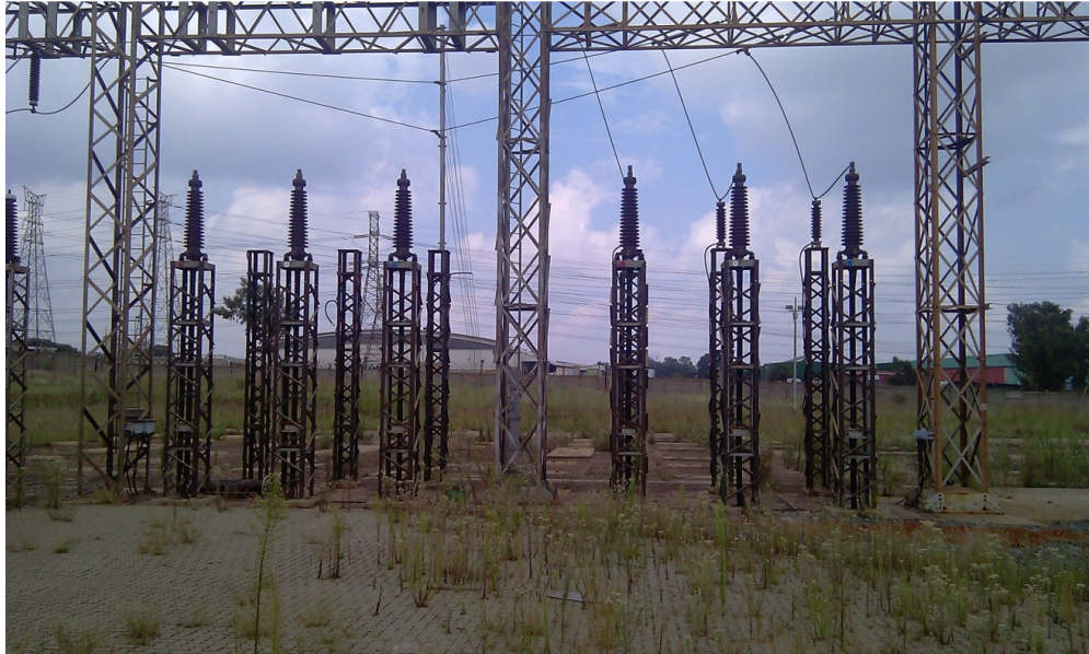
Spare 88kV bays available at Moffat Substation
