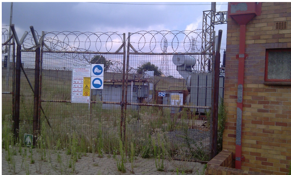
Space available on either side to extend the existing Substation
